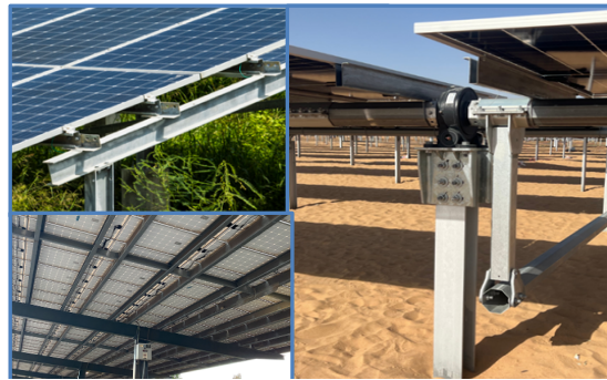
Figure 2 - Solar mounting systems and the many connections
