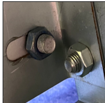
Image 4: Example of improperly designed or assembled bolted joint – missing washer.
