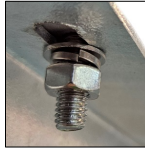
Image 31: Helical washer in a loose module through-bolted joint.
