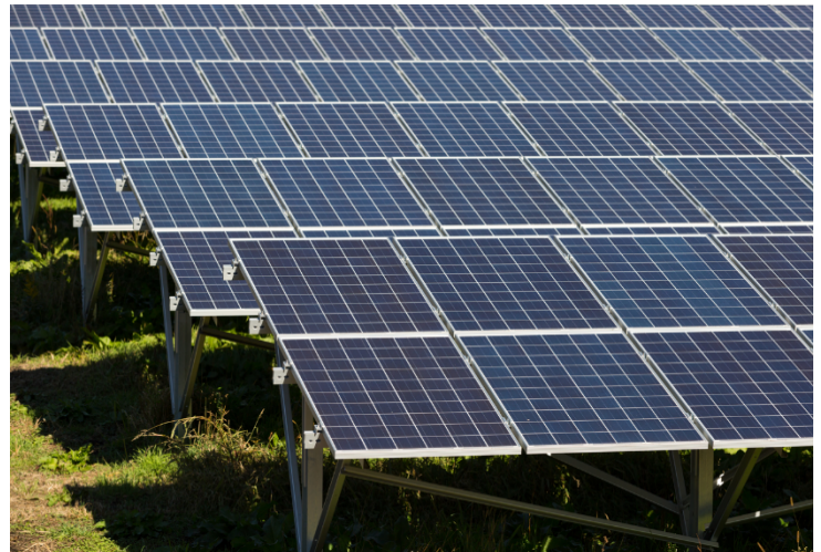
Figure 1: A typical utility-scale solar photovoltaic (PV) site consists of hundreds of thousands of identical mounting systems, each containing multiple bolted joints, amounting to millions across the site.
