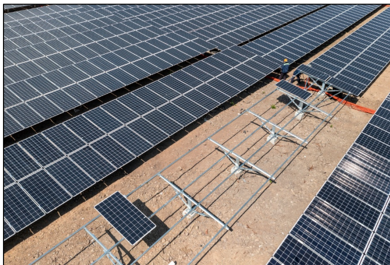
Figure 2: Typical utility-scale solar PV construction site. The bolted joints in the PV mounting systems are almost universally tightened using the torque control tightening method.
