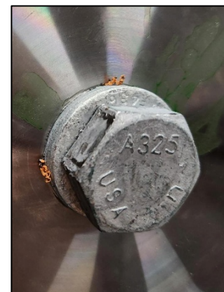
Figure 11: DTI washer with silicone indicators provides a visual clue that the minimum pretension has been achieved during tightening.
